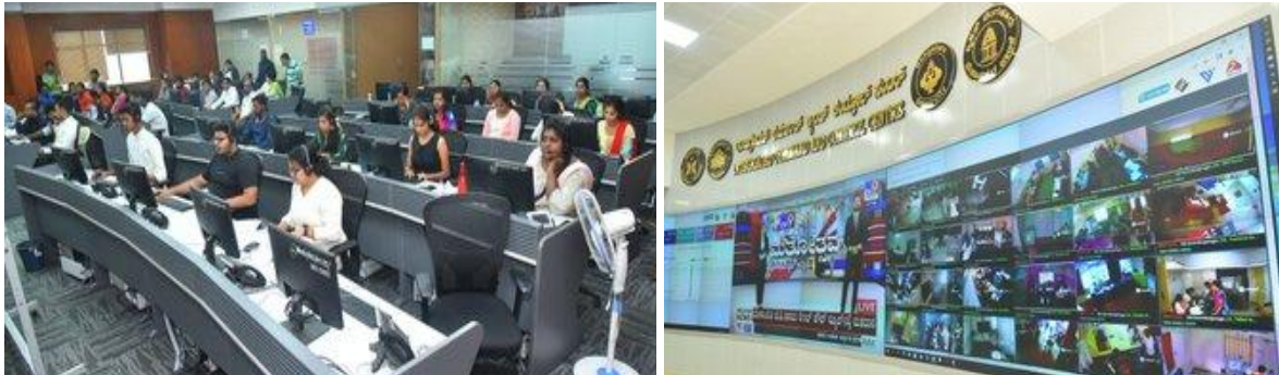
Integrated Control and Command centre at BBMP for monitoring of PS in 28 ACs
